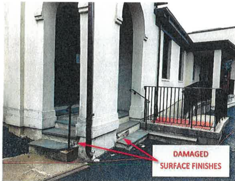
Photo 8 - Damaged Finishes Near Column Base
