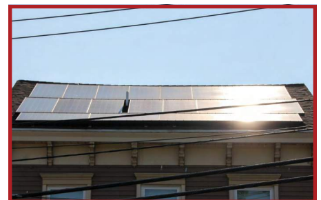
✗ Inappropriate Solar panels visible from primary frontage
